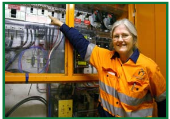
Manager, Chemical Processes, Helen Faber, in the existing switch room.
